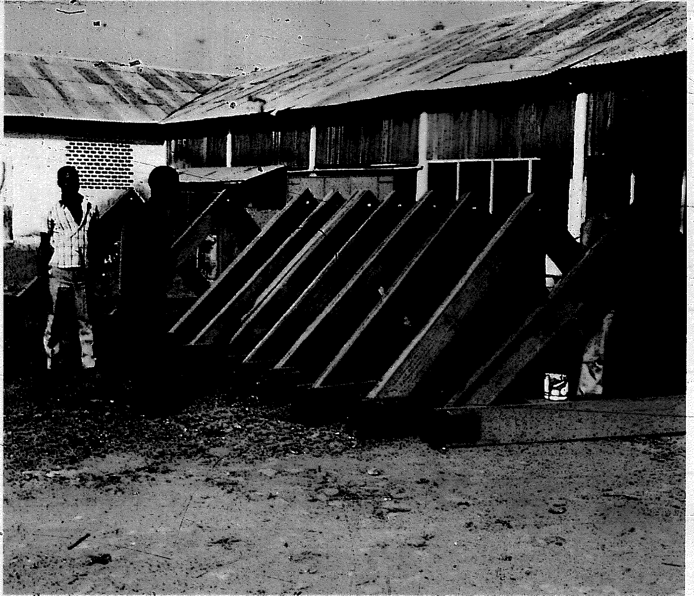
Panels and steel tension chords completed at the workshop await transport to the bridge site at Avakaba, Central African Republic
