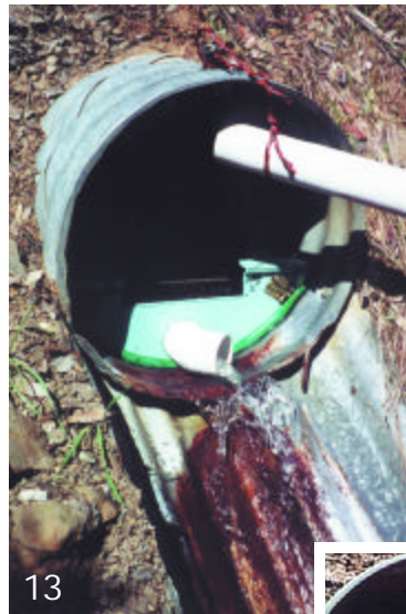
13. The diversion pipe from the culvert dam can be removed and tied off when not in use.
