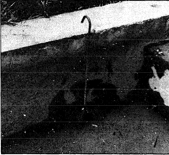
Fig. 5.174. This simple sliding gate is used when the settling basin is to be drained.
