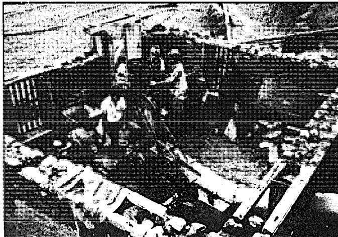
Fig. 10.20. At this new mill, no intermediate drive shaft is used between the turbine and agro-processing equipment.
