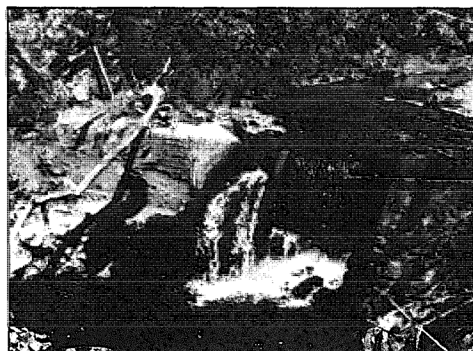
Fig. 5.39. Even before an opening for the penstock pipe could be made through the concrete intake structure to the left of the weir, flows had already seriously undermined the structure and completely backfilled the intake and area behind the weir. The design did not include an opening behind the weir for sluicing out the accumulated sediment behind it.
