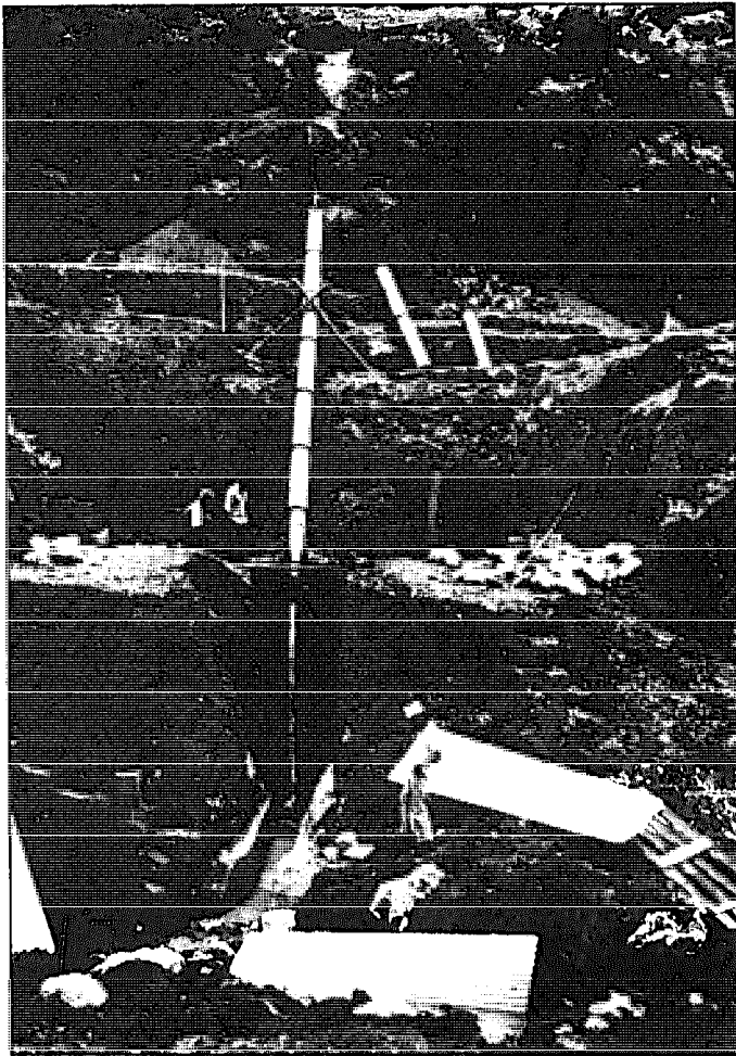
Fig. 10.26. The penstock, turbine, and draft tube are all assembled and properly aligned before they are set in concrete. A portion of the tailrace canal has already been completed.
