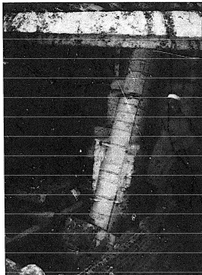
Fig. 10.57. The oil-drum penstock at the Alpuri powerhouse. The operator's bed is in the foreground.
