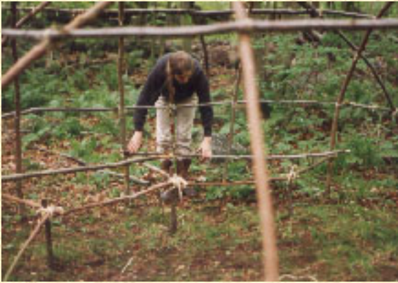
Again me, building the frame for the sleeping platforms inside the wigwam.
