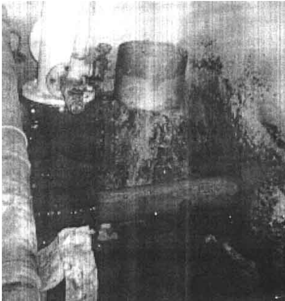
Fig. 6 RDTAC's Hydrum installed At Adami-Tulu
