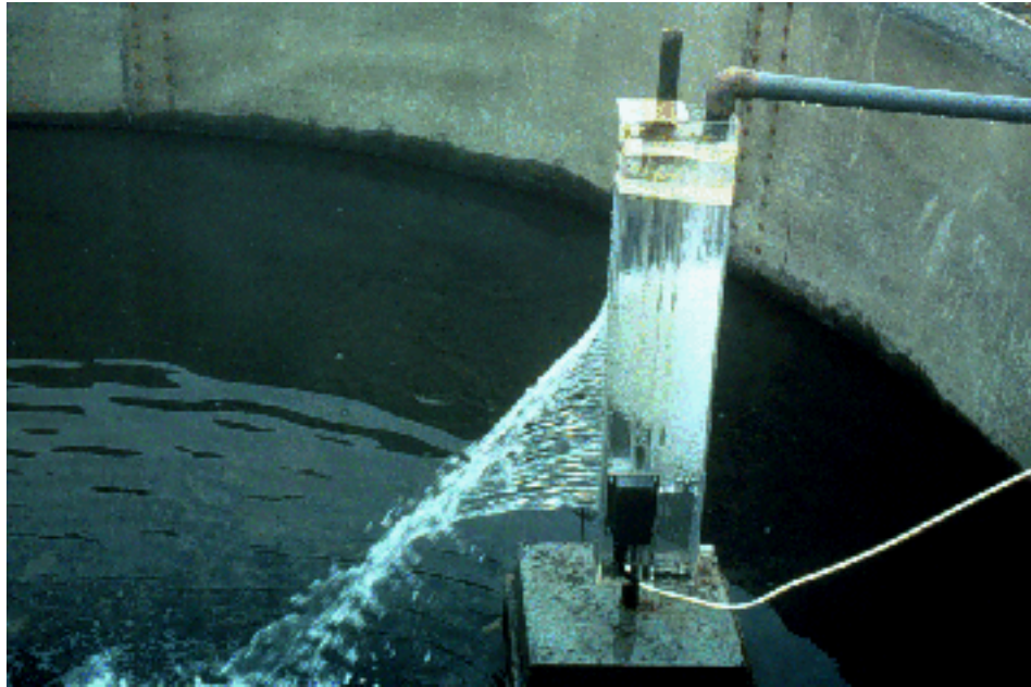
Fresh water flows into a storage tank
