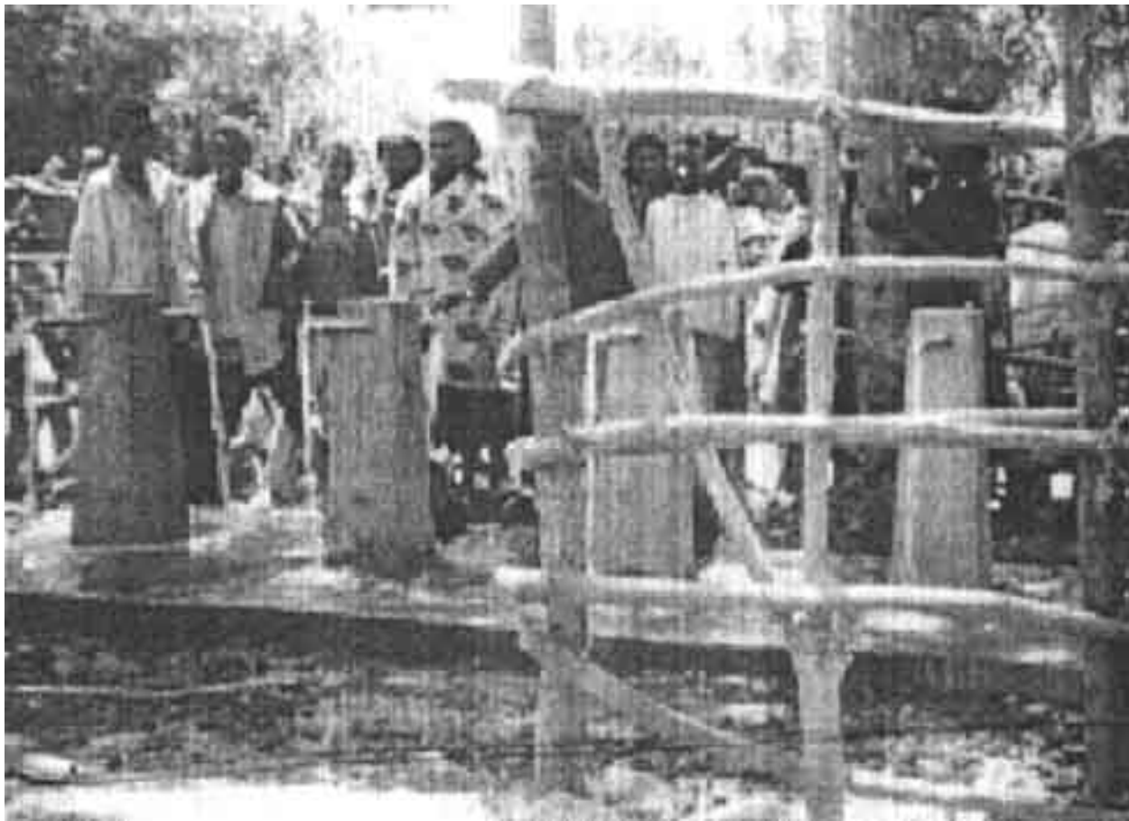
Fig.7 Water Supply System at Dodicha Woreda, Arsi Zone, Oromia Region from RDTAC's Hydram
