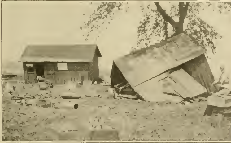
FIG. 3.—ANOTHER VIEW OF THE FLOOD DAMAGE
