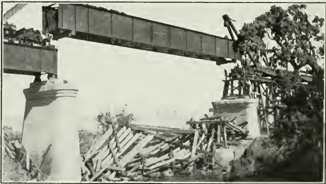
Fig. 3—Old Trestle Two Seconds after the Explosion
