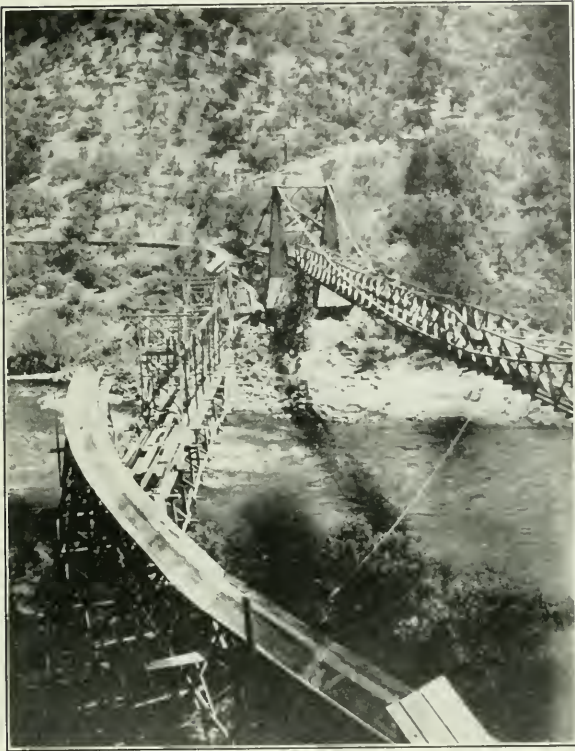
Old Suspension Bridge Across Kings River, California, on the Right; New Steel Bridge Under Construction, on the Left
