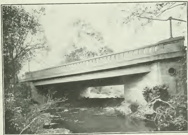
Fig. 7—Marsh Street Bridge, San Luis Obispo, California George Story, City Engineer John R. I. [unreadable], Consulting Engineer
