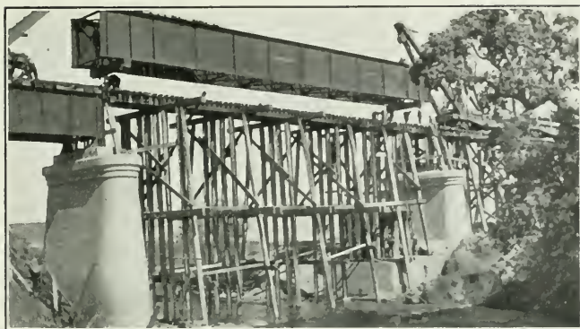
Fig. 1—Showing Steel Girder and Wooden Trestle Before the Explosion
