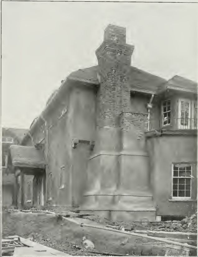
Residence of Mr. Mortimer Fleishhacker, Redwood City, California, After Being Treated With "Gunite"
