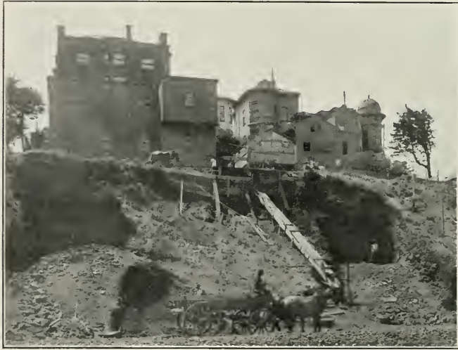
Site of Apartments for Mr. A. B. Hammond and Dr. L. Mace, San Francisco
