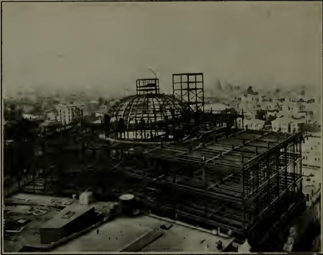
Steel Frame, Kahn Building, Oakland. C. W. Dickey, Architect Dyer Bros., Fabricators
