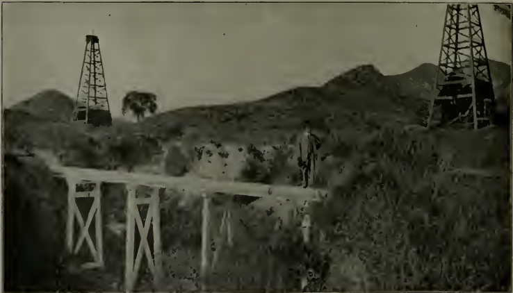
View of Corrugated Culvert Pipe Carried Over a Deep Arroyo on a Wooden Trestle Without Provision for Expansion and Contraction
