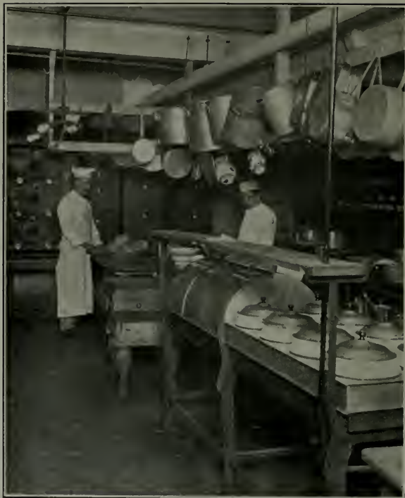
Electrically Equipped Kitchen, Stanley Hotel
