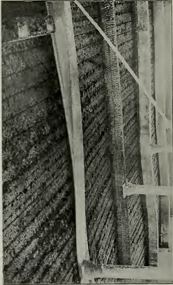
Wooden Timber vs. Unprotected Steel Beams. The stability of the single eight by ten inch wooden timber was not affected, although the ten inch steel beams sagged and were twisted to a degree which required rebuilding. The wooden beam was used because not enough steel had been ordered to complete the work promptly. In rebuilding, wooden beams were used throughout.
