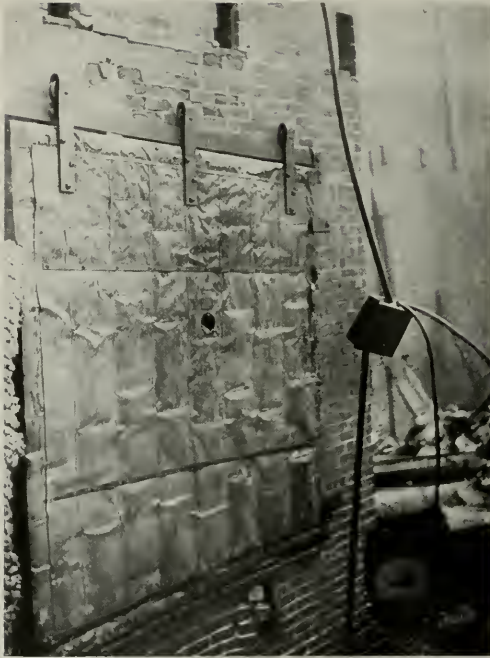
A Standard Fire Door. —In a large paper warehouse in which everything in one section was destroyed by fire, a line of standard tin-clad fire doors effectively protected all stories of the adjoining section. The accompanying photograph shows one of the doors. Self-releasing timbers saved the walls from wreck, and the doors kept the fire in the burning section. Note the integrity of the standard hardware and the unwarped body of the door due to its well selected lumber and proper nailing. Nothing happened to it but the bite the fire took out of the core exposed in the little round gas-vent.
