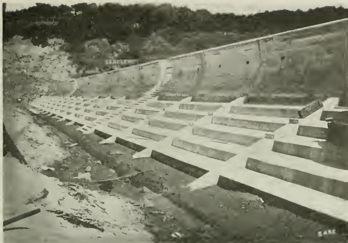
COMPLETED SECTION OF OCEAN BEACH ESPLANADE, SAN FRANCISCO M. M. O'Shaughnessy, City Engineer
