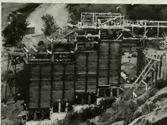
Part of an #1 & #6 Rock and Gravel Plant
