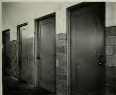
Detail of five-foot wainscoting of Kraftile 6x9's at doors of service rooms of Fresno fire department headquarters. The tile is stain-proof, acid proof and easily cleaned. The larger size of tile facilitates the wainscots design.
