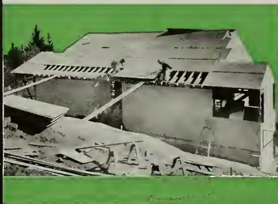
On this Portland, Oregon, home, 5/16" Plyscord was used as wall sheathing, 3/8" as roof sheathing and 5/8" as sub-flooring. (The 5/8" Plyscord was used first as concrete form material.) This house is 40% more rigid than if diagonal board sheathing had been used. Cutting, fitting and nailing were minimized. The 5/8" Plyscord sub-floor, for example, went down in just half the usual time. Richard Sundeleal was the architect.
