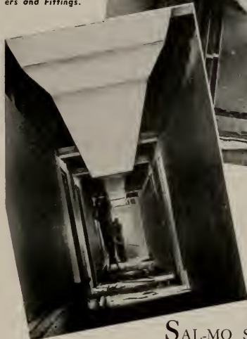
A Typical Installation of Sal-Mo Supply Duct in a Defense Housing Project.
