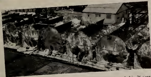
WRECKS ASPHALT PLANT TO GET WAR SCRAP - Demolition of this 26-year-old asphalt plant by an eastern refining company is yielding over a thousand tons of precious scrap, enough to make the steel for 70 "General Lee" tanks. . . . Do you have any steel structures, idle now and of doubtful future value, which should be wrecked to release the scrap metal they contain?
