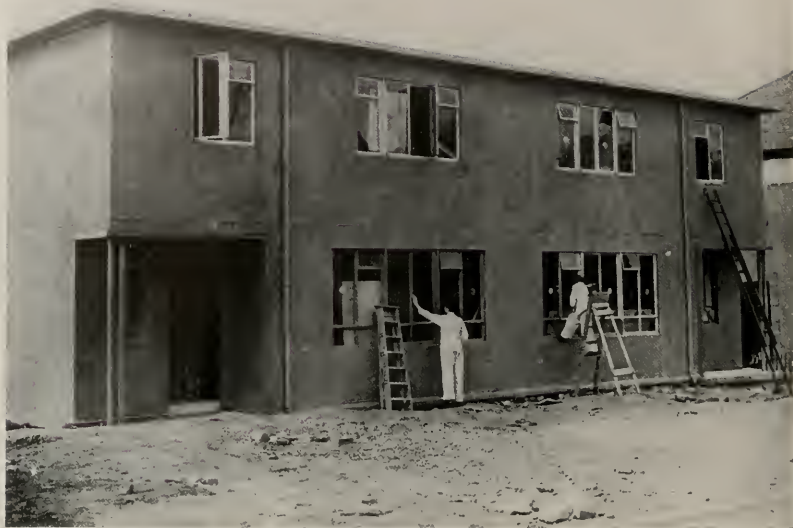
FIRST WEIR STEEL PREFAB SEMI-VILLA. Painters line off window frames and put the finishing touches to the first Weir steel house in Knightswood, Glasgow.
