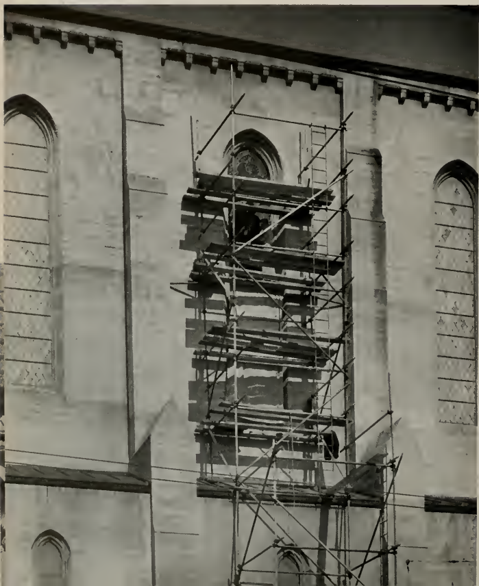
The installation of a window of this size presents a problem of scaffolding. The peak of this window is 75 feet from the ground and the scaffolding is set in sections and levels to enable easier installation.
