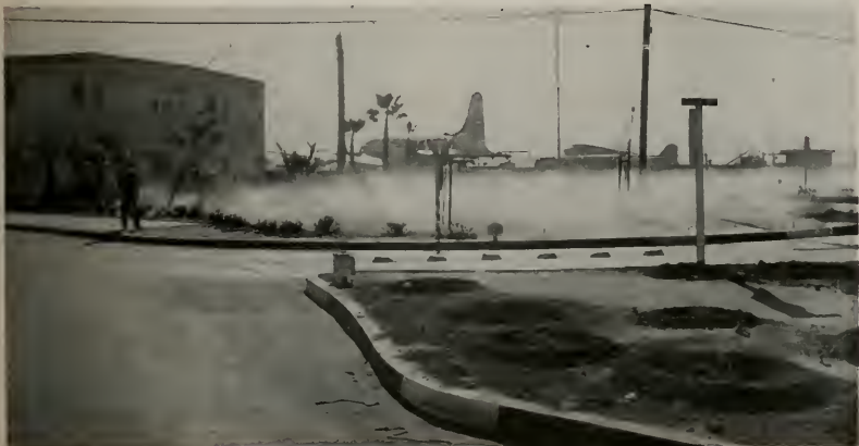
Sprinkler system in operation. View shows parts of three planted areas with the island at the left planted with Gelsemium as a ground cover. Los Angeles Airport.
