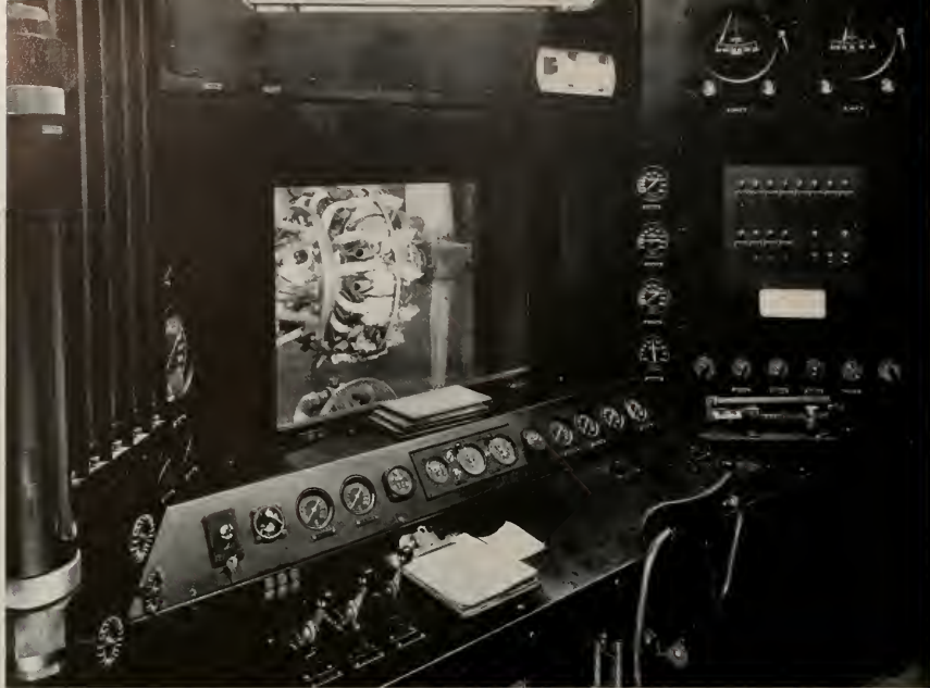
All of the operating controls and metering devices required for engine testing in the new "test cells," are grouped around double-glazed observation windows in compact and convenient arrangement. Six control desks, similar to one illustrated above, are paired in the control passages extending through the cell block. Sperry controls (left foreground) and potentiometer is mounted flush on desk at right with slant gauge directly above window. Engine in position for testing is seen in test cell.
