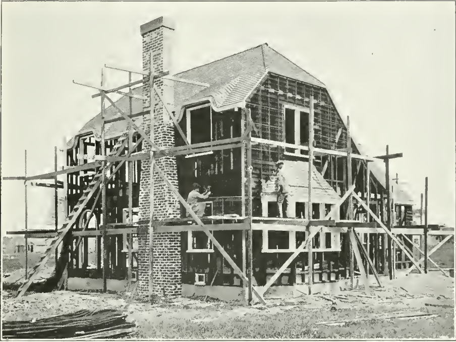
RESIDENCE, STOCKTON, CALIFORNIA. LOSEKANN & CLOUDSLEY, ARCHITECTS Showing Application of Metal Lath Direct to Studs Without Sheathing Boards.
