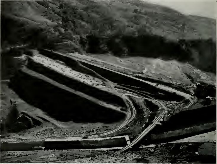
CALAVERAS DAM CARRIED TO A HEIGHT OF 215 FEET ABOVE ITS FOUNDATION, SHOWING BERM CONSTRUCTION OF THE DOWN-STREAM SLOPE
