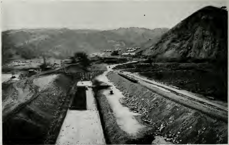
ROLLED CLAY CORE OF CALAVERAS DAM UNDER CONSTRUCTION. THIS CORE IS SUPPORTED BY THE EMBANKMENTS OF ROCKY MATERIAL
