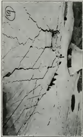
SAGGING OF CONCRETE FLOORS
