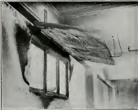
NOTE COLLAPSED WIRE GLASS AND EFFECTS OF HEAT ON THE SHUTTER
