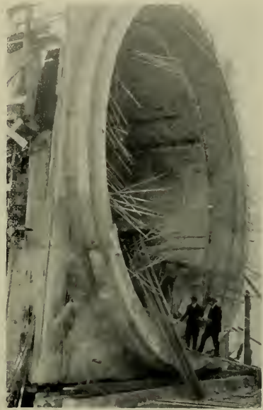
END OF COMPLETED CONCRETE SEGMENT Showing Collar and Inside Joint Lap Reinforcement
