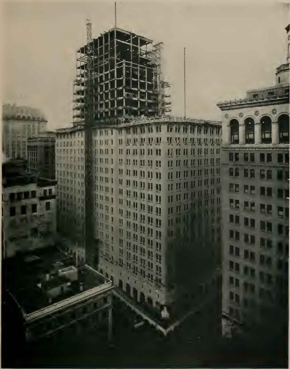
RUSS BUILDING, SAN FRANCISCO. GEORGE W. KELHAM, ARCHITECT SHOWING ABOUT TWO-THIRDS OF ITS 30-STORY HEIGHT
