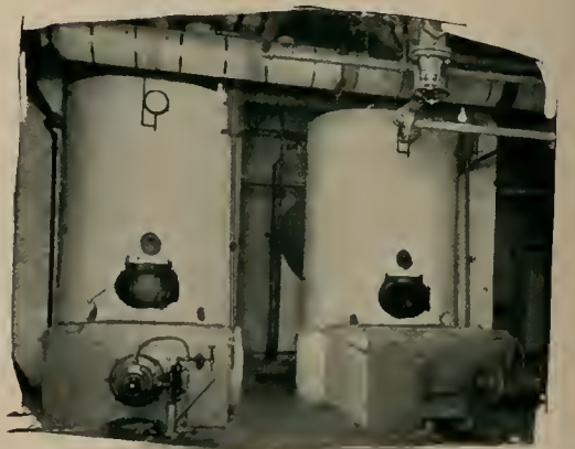
Oil Burner Installation by Fuel Oil Burner Engineering Co., New York City.
