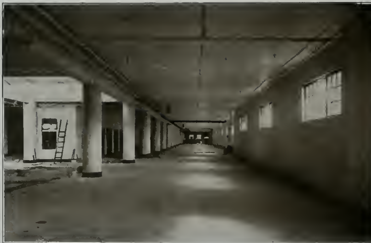
Metal Lath and Plastered Ceiling—Meyer System Floor Construction MAY CO. DEPARTMENT STORE, CLEVELAND, OHIO Graham, Burnham Co., Architects
