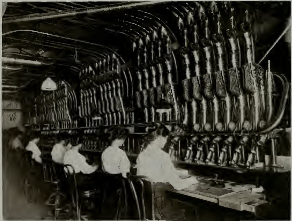
Section of Convergence of Cash Tubes MEIER AND FRANK CO. BUILDING, PORTLAND Doyle & Patterson, Architects
