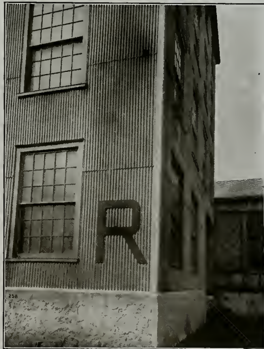
Ambler Corrugated Asbestos Used as Siding with Ambler Flat Asbestos Building Lumber for Framing, and Asbestos Ridges Roll on Corners. Neighboring Building Covered with Century Asbestos Shingles
