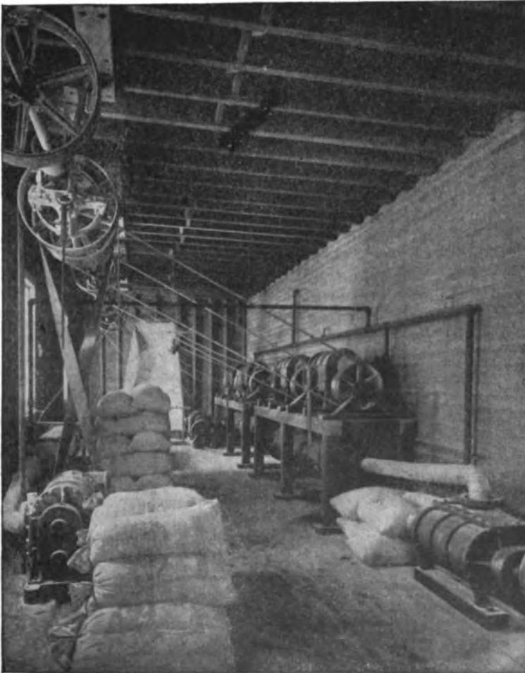
Fig. 117.— Blowers and Air Sterilizing Apparatus.
