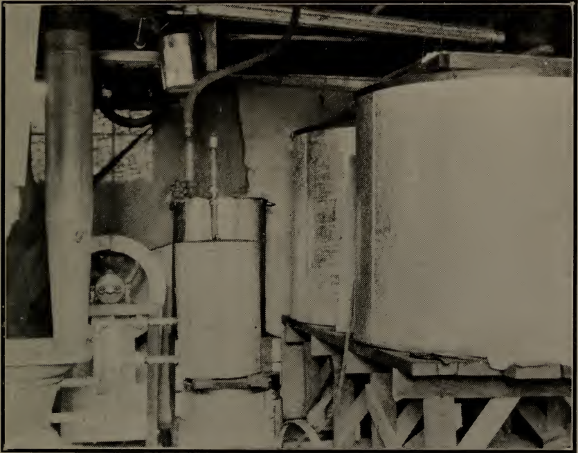
Fig. 61. Settling tanks and heating system are in the basement of the Sutton central plant.
