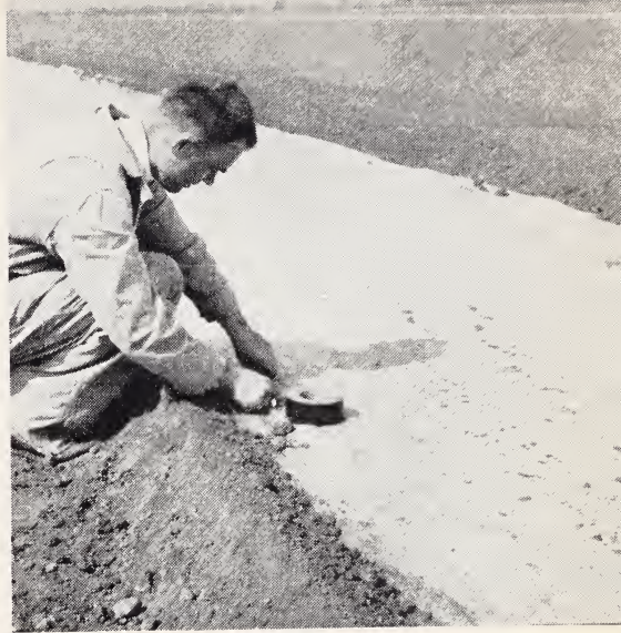
Fig. 7. All rips in the polyethylene, even minute rips, must be patched, and if strong winds are a threat the covered areas must be patrolled for blowouts.
