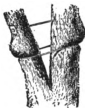
FIG. 155. — A good and a bad way to strengthen a weak crotch of a tree. Better yet, in many cases, is the use of a chain between two bolts instead of the single long bolt. (From Bailey.)
