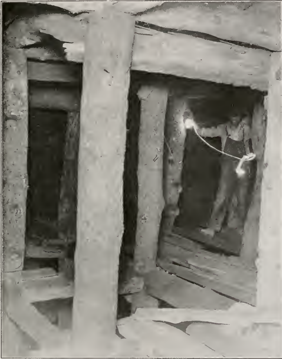
Photo No. 22. Flashlight view in square set stope (30' wide) between No. 2 and No. 2½ levels, New Idria Mine.
