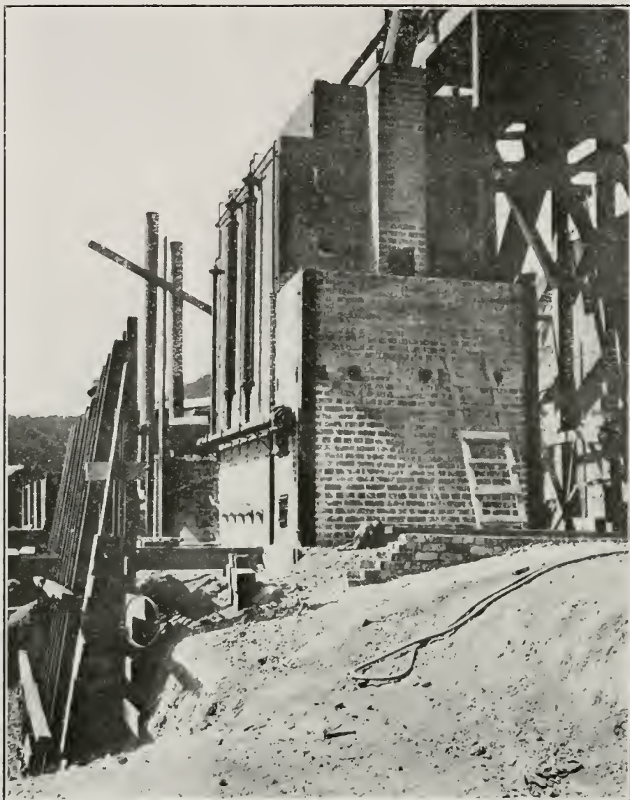
Photo No. 45. Livingston Furnace under construction at La Joya Mine, Napa County.
