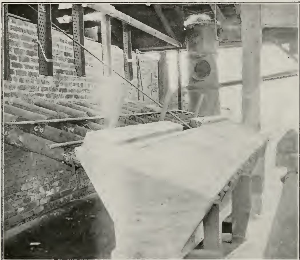
Photo No. 63. Condenser System on Johnson-McKay Retorts at Sulphur Bank Mine, Lake County.
