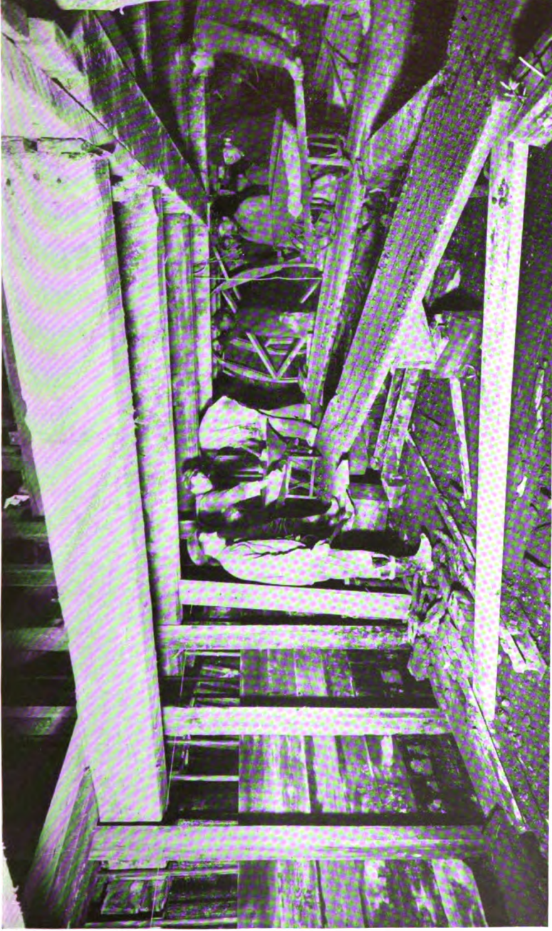
PLACING CONCRETE IN FORMS FOR WALLS OF REINFORCED CONCRETE WAREHOUSE FOR STEEL-WEDELES CO., CHICAGO, ILL.
