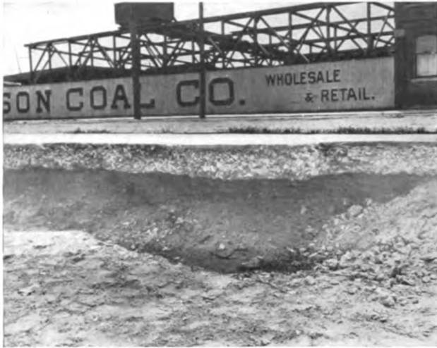
RESULT OF INSUFFICIENT FILL FOR CONCRETE SIDEWALK.
