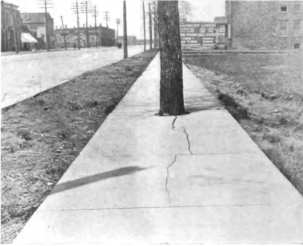
CRACK IN CONCRETE SIDEWALK CAUSED BY TREE.
