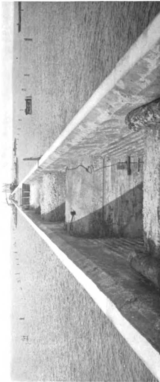
LONG KEY OCEAN VIADUCT ON KEY WEST EXTENSION OF FLORIDA EAST COAST RAILWAY.
