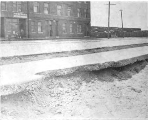
RESULT OF NOT PROTECTING THE EDGE IN LAYING CON- CRETE SIDEWALK.
