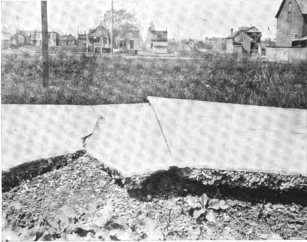
CONCRETE WALK DESTROYED BY EXPANSION.
