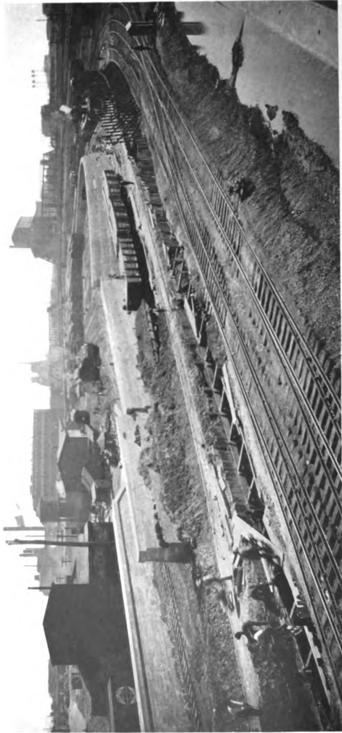
PART OF MORE THAN 1,600 MILES OF STEAM RAILROAD TRACK IN COURSE OF ELEVATION IN CHICAGO, ILLINOIS.
