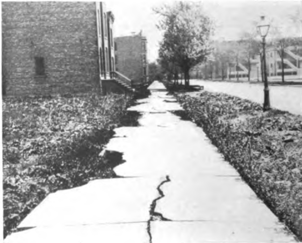
RESULT OF LAYING SIDEWALK DIRECTLY ON THE GROUND.
