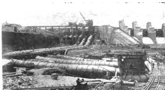
FIG. 3b. The penstocks of the Gatun plant. The water turbines in the process of erection. The Electrical World.
