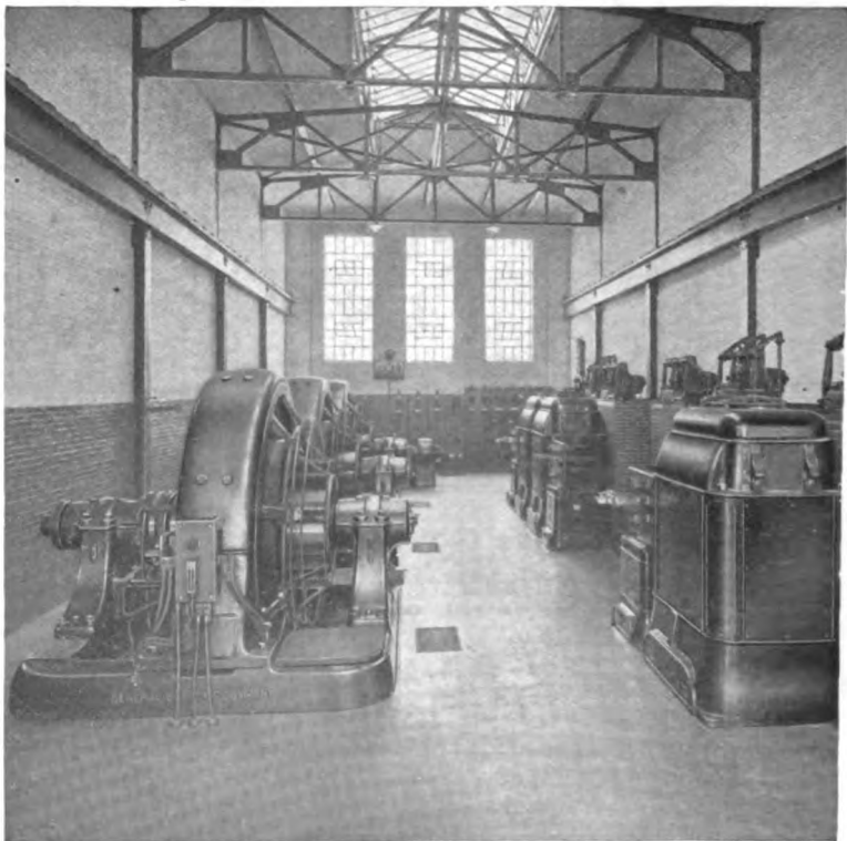
FIG. 7c. A converter substation containing synchronous converters. Note that no separate motor is required to drive such a converter. The General Electric Co.
