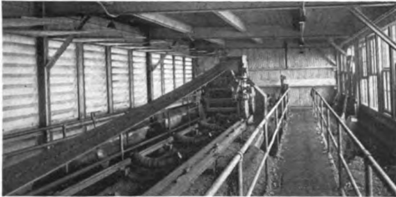
FIG. 1b. A coal conveyor for delivering coal to the hoppers above the boilers. The Electrical World.
