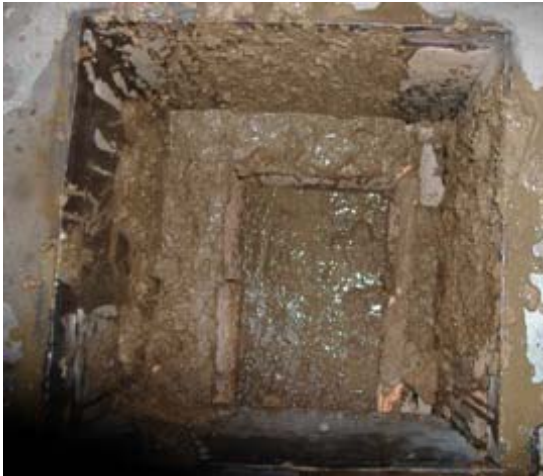
Photo 30: Using grog to bind the combustion chamber box with the liner
