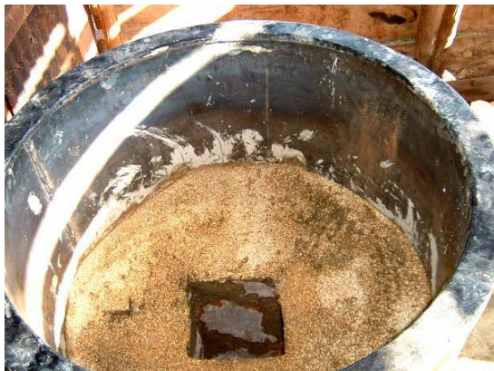
Photo 31: The inside of a chamber with an insulation slant set onto the base plate
