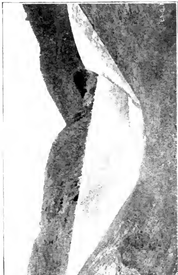
Fig. 146. Concrete-Lined Section of Truckee Canal, Nevada. Junction of earth and concrete-lined section, showing warped surface in latter.
