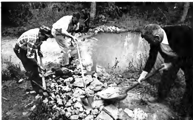
"U.S." employees, such as the above, tackled the forbidding terrain and details of the construction. Things moved quickly!
