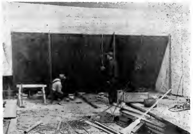
Underground water basin in an unused city water plant gets converted into rifle range for recreation and police use.
