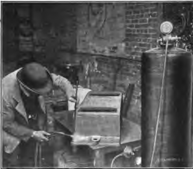
Fig. 5. Welding the Broken Flange of a Cast-iron Base. The Operator feeds the Joint with a Cast-iron Rod
