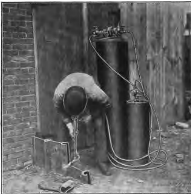
Fig. 6. Cutting Off Steel Sheet Piling with Oxygen Cutting Torch showing Portable Apparatus
