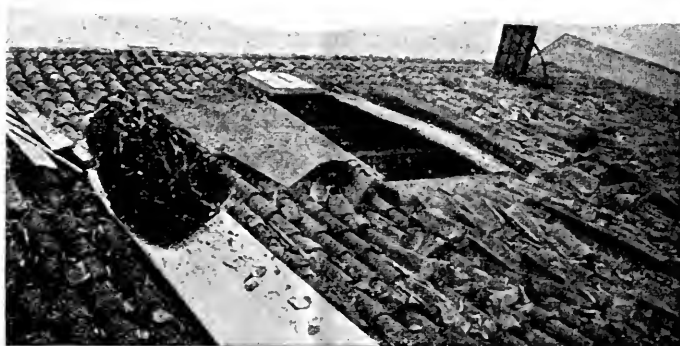
FIG. 3. THE DAMAGED ROOF, SHOWING FRAGMENT OF GENERATOR FRAME.
