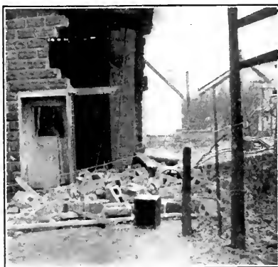
FIG. 1. WRECKED BOILER HOUSE.
