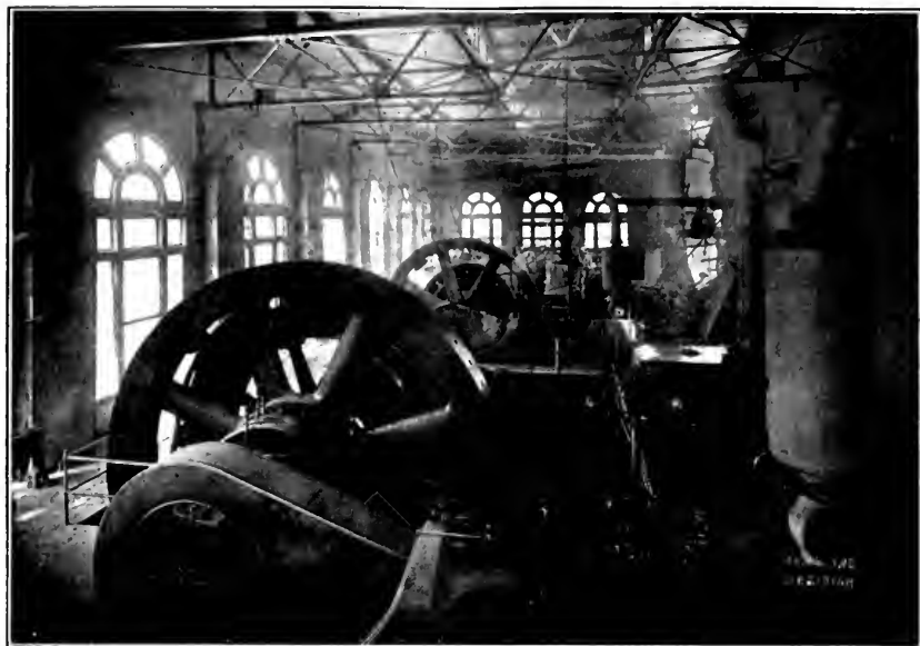
FIG. 3. WRECKED ENGINE AND TURBINE ROOM.
