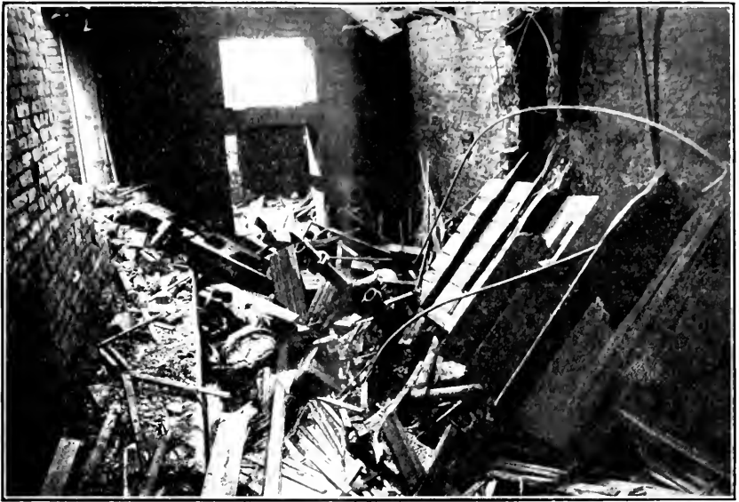
FIG. 2. WRECKED BOILER ROOM AT ST. JOHN'S CHURCH.
