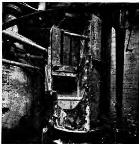
WRECK OF AN OPEN FEED WATER HEATER.
