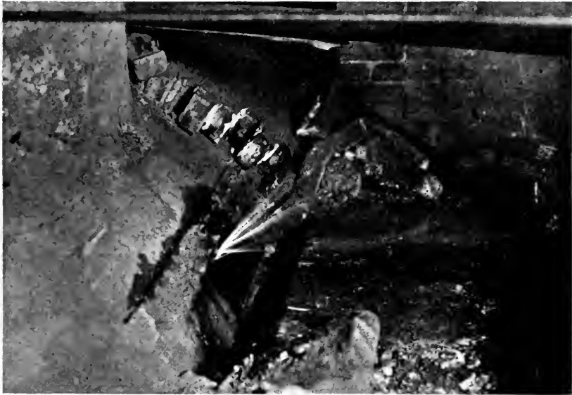
WATER ISSUING FROM A LAP SEAM CRACK.
