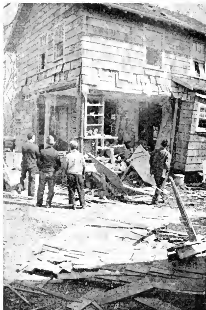
After a hot water tank exploded.
