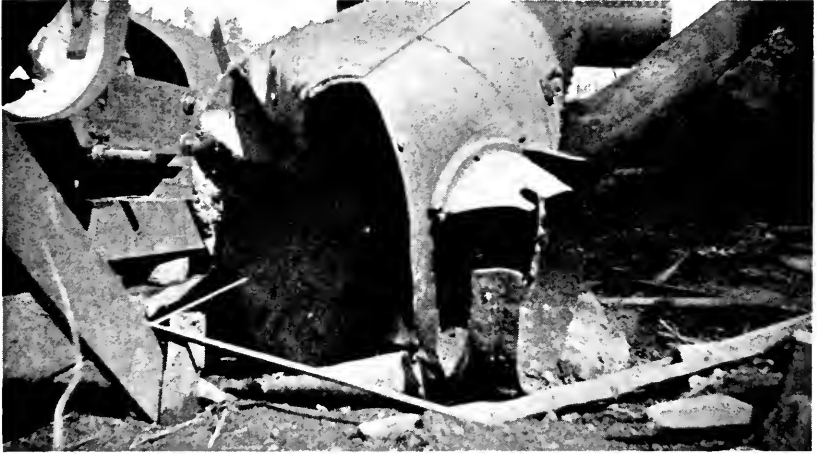
Figure 2. Aftermath of corrosion around the crown bolts of a locomotive type boiler.
