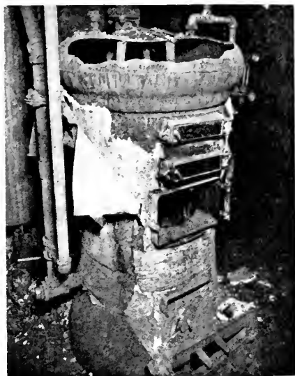
Figure 2. Partial damage following a cast iron boiler explosion.
