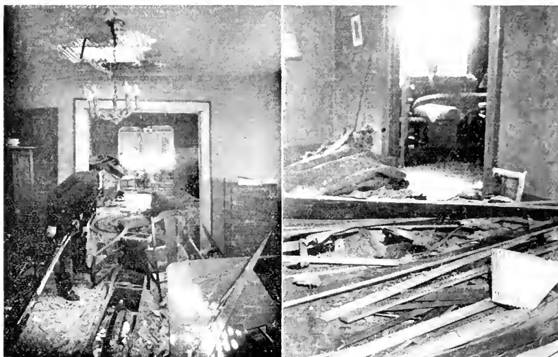
After hot water tanks hurtled upward.
