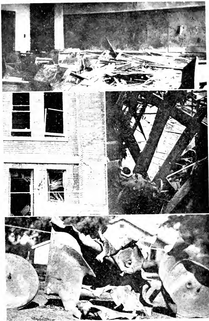
Scenes at Forest, Mississippi. Top and right center—pieces of the school-room floor. Left center—cracks in the building. Bottom—pieces of the tank.
