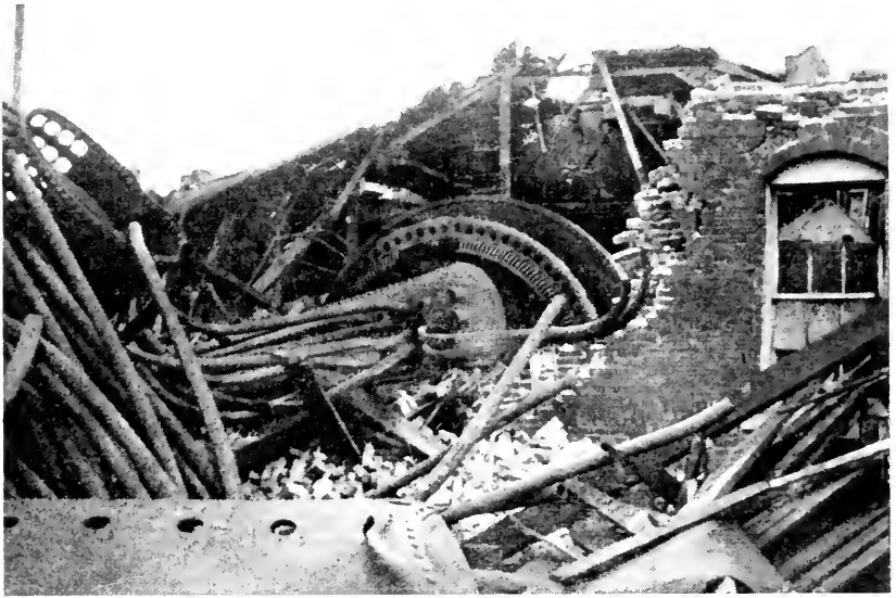
Wreckage following a lower drum failure at a Middle-Western utility.
