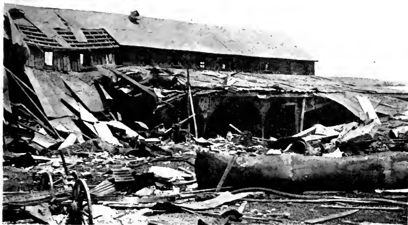
Figure 1. Result of a lap seam failure early in June.
