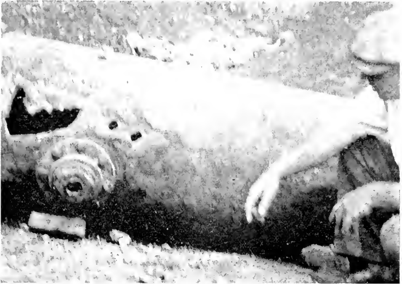
Extreme external corrosion in a buried blow-off tank. Conditions with respect to this form of wasting away are particularly serious whenever a vessel is installed underground.
