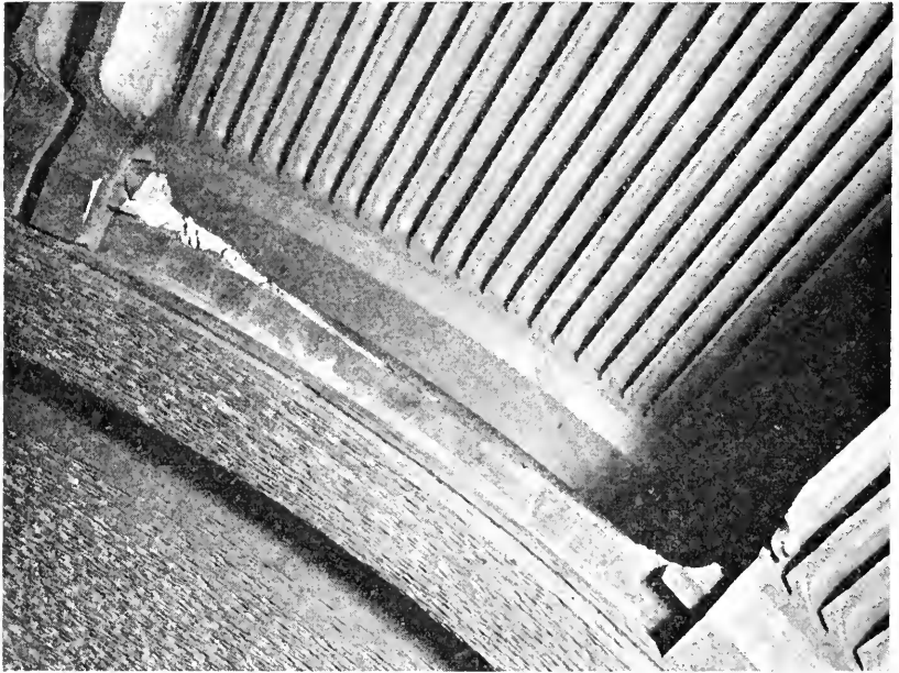
Figure 1—The broken disc. The dovetail arrangement of fastening the blades is clearly visible at the left.
