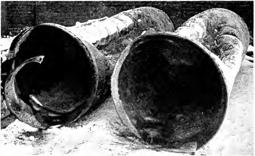
Collapsed Scotch-Marine boiler furnaces, the result of overheating.
