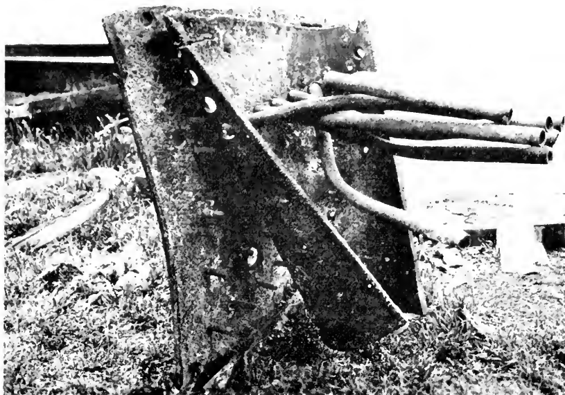
Once part of a hot water supply system.
