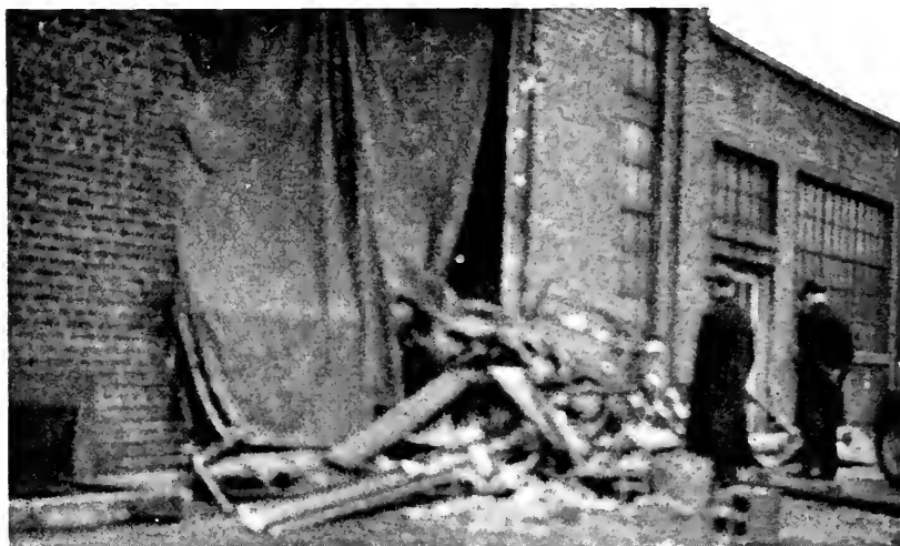
Damage caused by the explosion of an open type feedwater heater.
