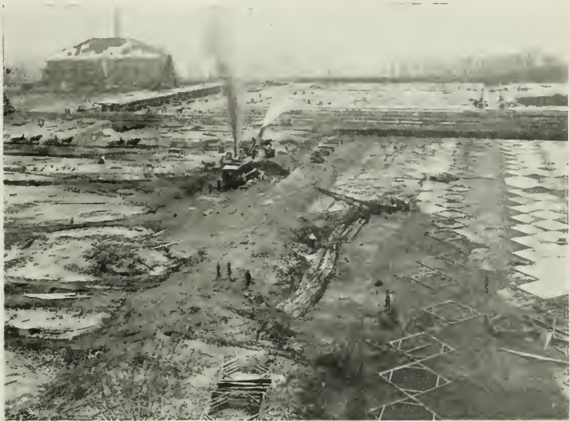
Fig. 47. Birds-eye View of Sedimentation Basin under Construction. Showing Ross Pumping Station in the Distance.
