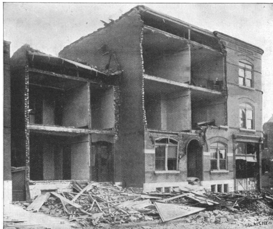
FRONT WALLS FORCED OUT BY VACUUM WITHOUT. LAMP LEFT STANDING ON TABLE ON SECOND FLOOR.
