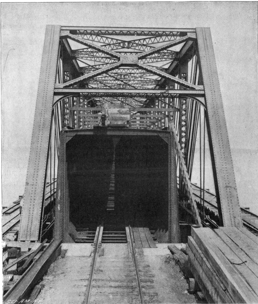
VICTORIA JUBILEE BRIDGE—END VIEW, SHOWING PIN-CONNECTED STRUCTURE ERECTED AROUND THE OLD TUBULAR BRIDGE.
