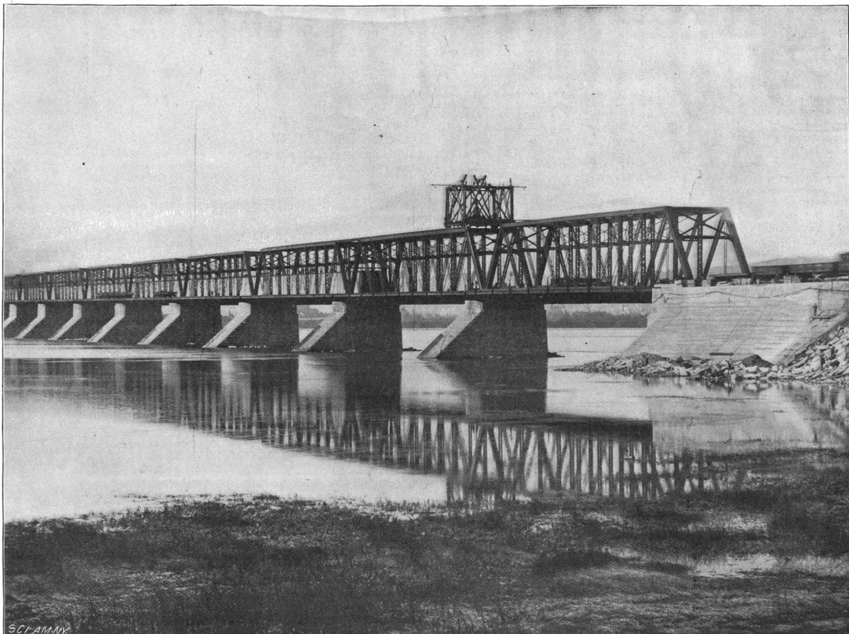
THE RECONSTRUCTION OF THE VICTORIA TUBULAR BRIDGE—VIEW FROM EASTERLY SHORE, SHOWING OLD TUBULAR BRIDGE IN COURSE OF REMOVAL.
