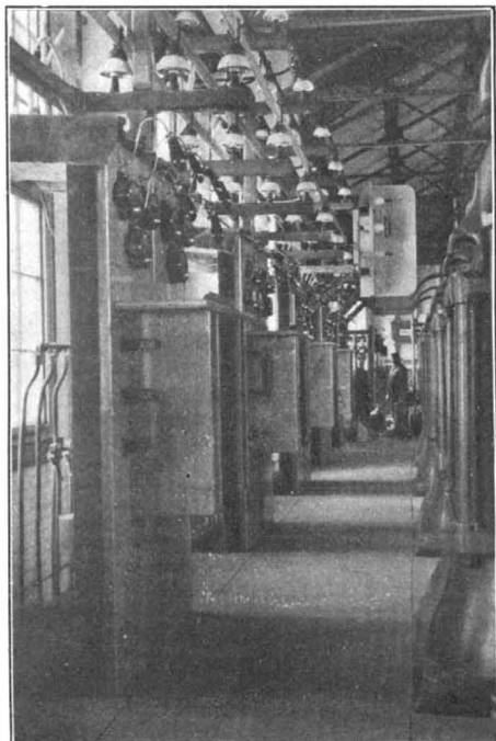
1.—High Potential Panels for Transformers.
