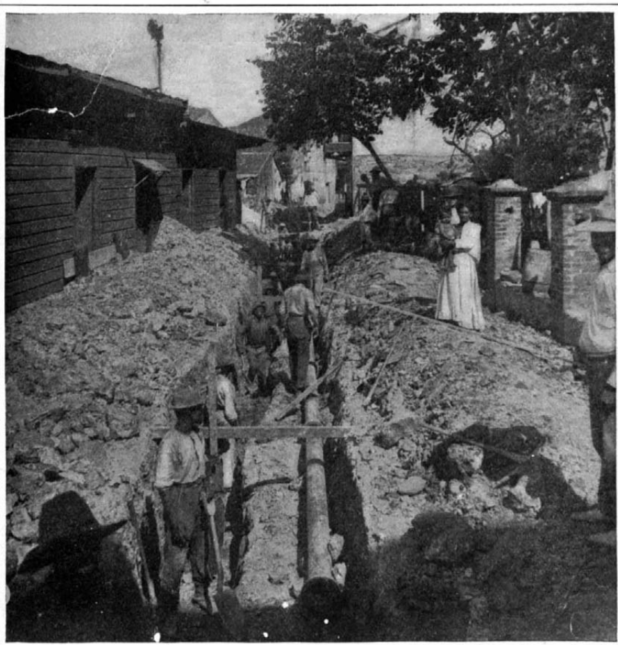
Laborers Excavating for New Water and Sewer Service. Work Done Under Department of Municipal Engineering of Canal Zone.
