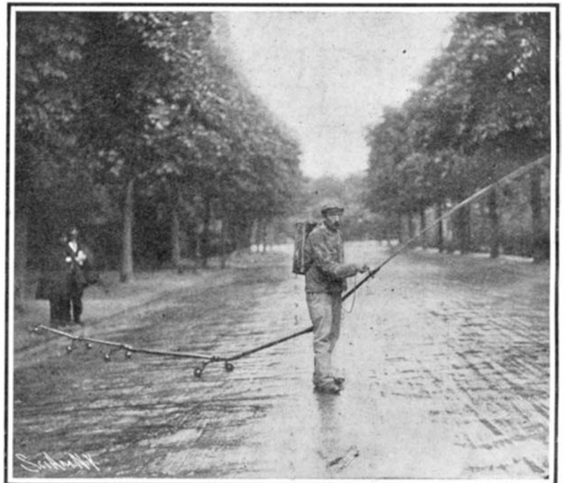
One Way of Applying Tar or Oil Consists in Piping the Water from the Mains Through a Hose. Oil or Tar is Fed to a Special Nozzle and Mixed with the Water.
