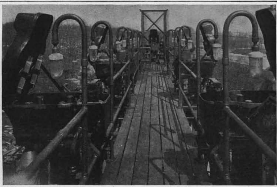
Set of Section Break Switches Shown in the Open Position.
