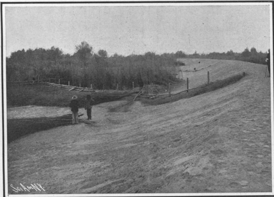
Partly Completed Portion of Yuma Levee, Showing Brush Work Constructed Along the Levee.
