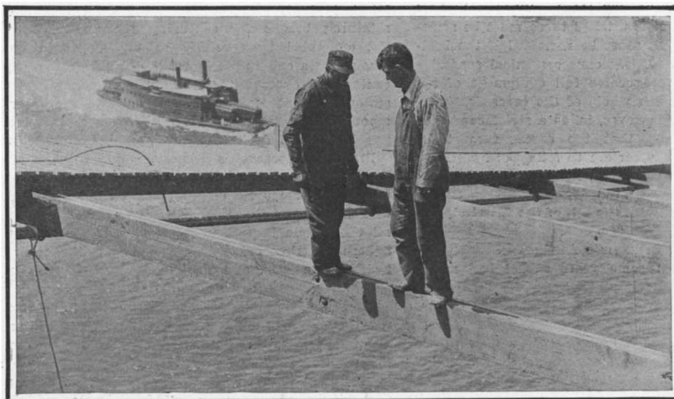
The Two Men Are Standing on a Pair of the 6 x 12 Inch Floorbeams Which Support the Footways. They Are 155 Feet Above the River.
