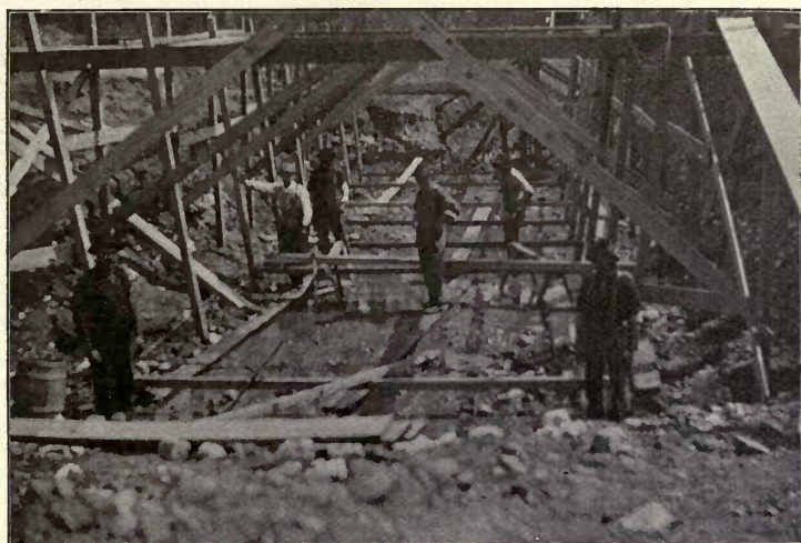
View of construction of Septic Tank at Wauwatosa, Wis. Framing of forms for concrete work.
