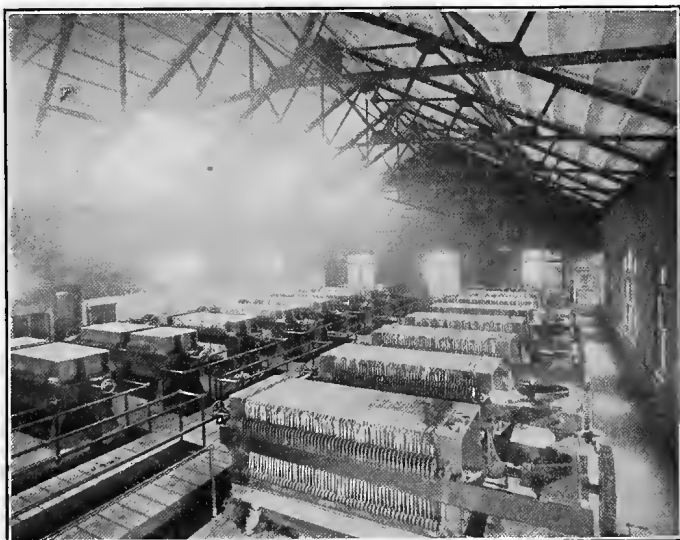
FIG. 40.—Sludge presses, Providence. (Courtesy of Mr. O. F. Clapp, City Engineer.)
