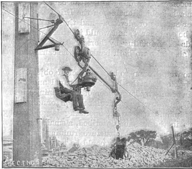
FIG. 71a.—THE LAMB ELECTRIC CABLEWAY.
