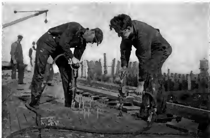
Fig. 97. The Pneumatic Hammer Driving Deck Spikes in Holes Which Have Been Drilled and Countersunk at the Same Operation by Another Little David. These Tools Make Short Work of Numerous Tasks
