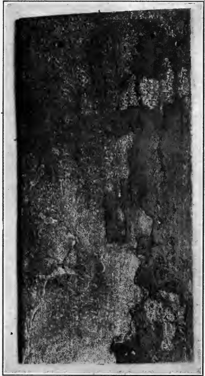
FIG. 298. — CORRODED STEEL PLATE.
