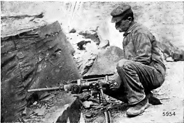
FIG. 15.—“Jack-hammer” at Work Drilling Horizontal Holes at the Diamond Slate Company’s Quarries, Pen Argyl, Pa. (Ingersoll-Rand Company.)
