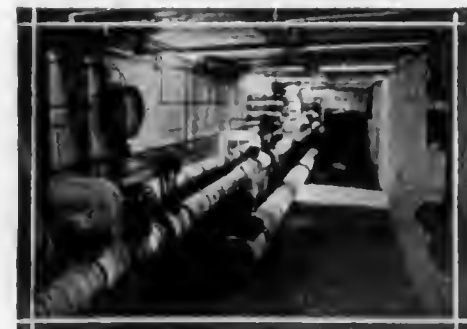
Operating pit which houses controls for coils and sprays.
