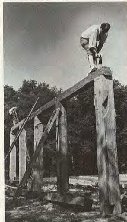
Carpenters at Carter's Grove plantation work on a seventeenth-century style tobacco barn.
